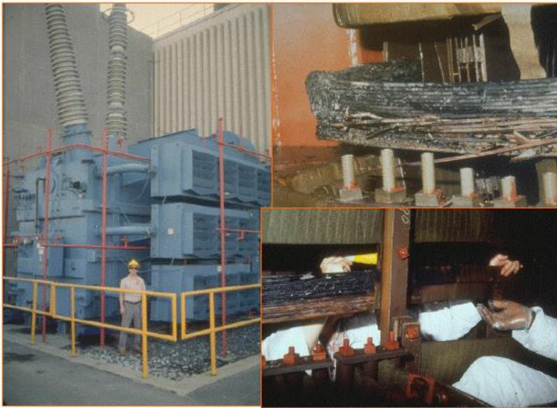
Figure 2-33. Damaged transformer at the Salem Nuclear Plant.
